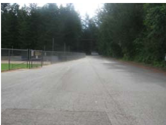
Leaves & Debris Frequently Clog the South Parking Lot Catch Basin
